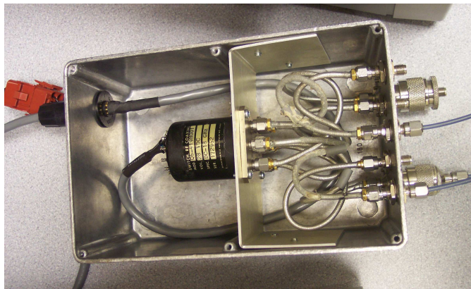
Figure 3.14: Weather resistant metal box containing the coaxial switch and associated cabling for the calibration update system.
